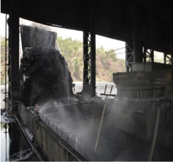
Automatic water spraying at crusher of CHP
